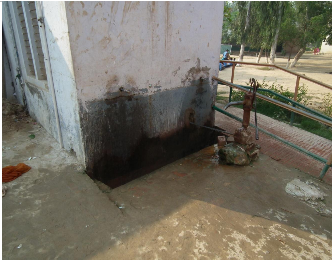
POOR CLEANLINESS OF DRINKING WATER AREA IN GSSS, DHARAMPURA
