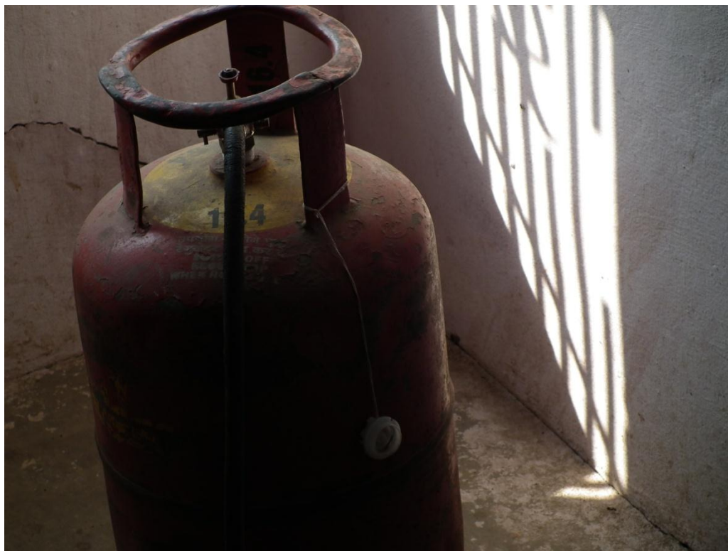
NON STANDARDISED GAS REGULATOR AND PIPE IN GES, JILLA JAIL, FARIDKOT
