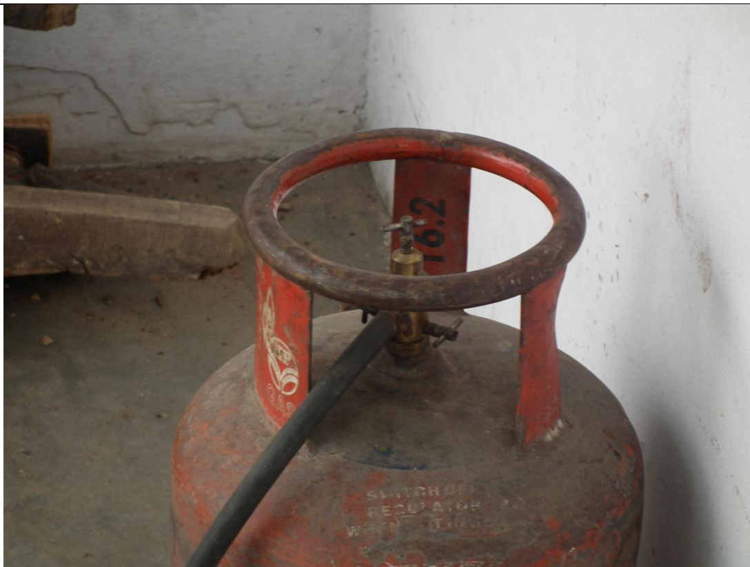
USE OF NON STANDARDISED GAS REGULATOR IN GHS, CHAJJALWADI
